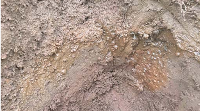
Figure 7. Water seepage from above compacted soil layer
